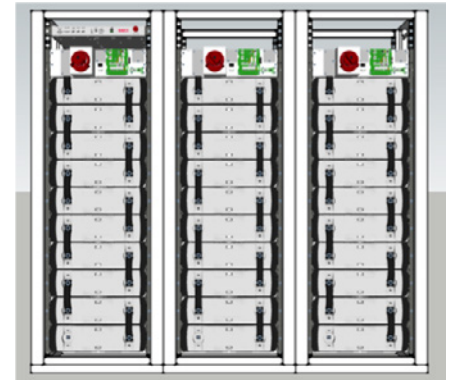
3 cabinets, 1 MBMM, 3 BMM, 10 Saft Synerion 48 V (in series) Example: typical 480 V Intensium® Flex 3 x 480 10.48P system, with 3 parallel strings (with 1 MBMM added to allow paralleling)
